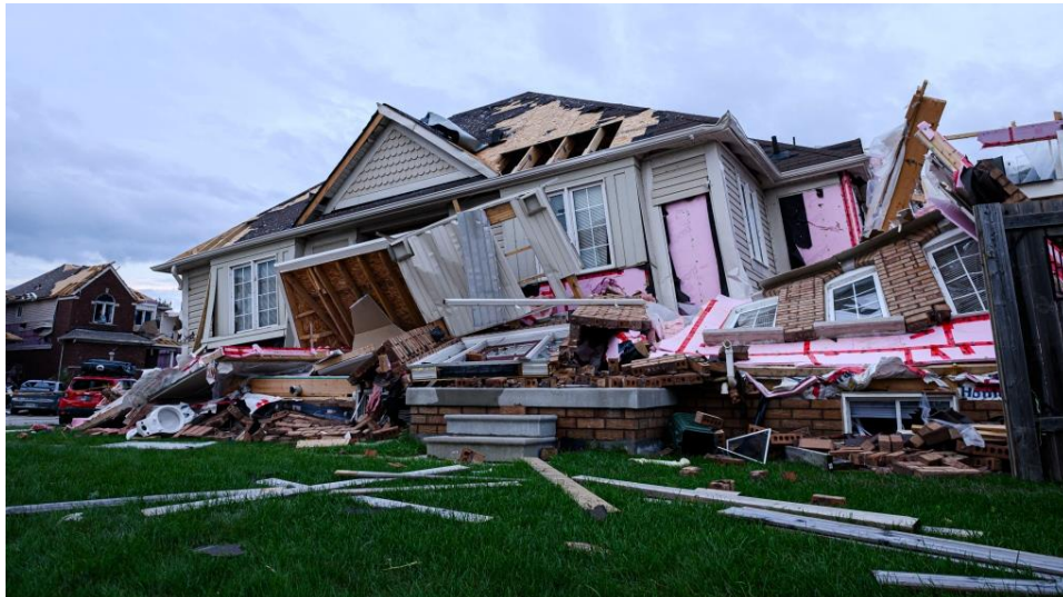
Damage from Barrie Tornado 2021
