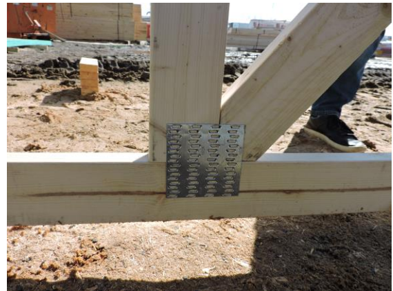
4x4 plate installed in the wrong orientation
