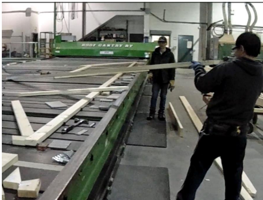
Worker checking the crook to make sure crown is up and flipping board
