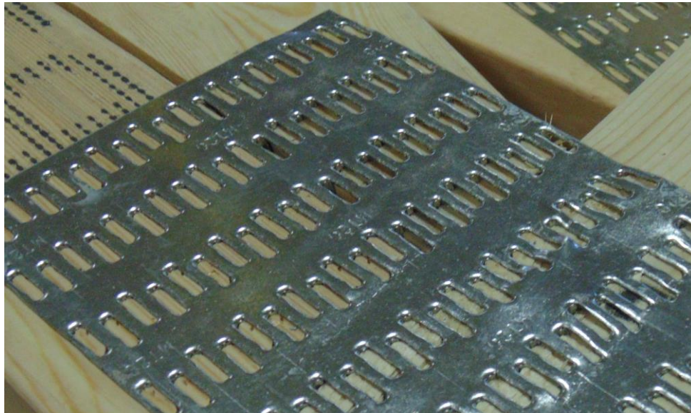
Embedment Gap in the web member
