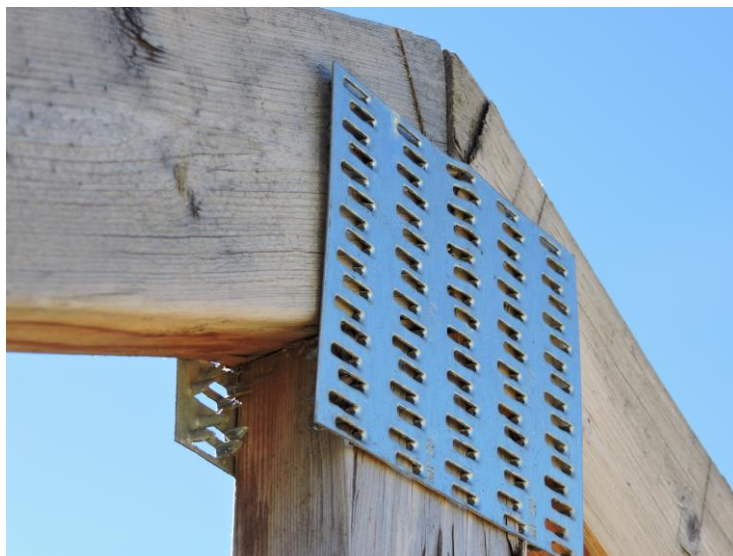
Trusses exposed to the weather causing lack of embedment
