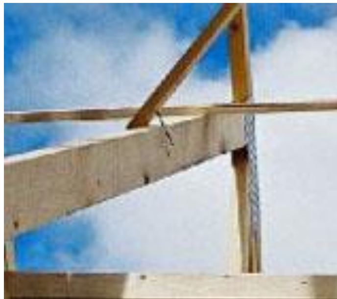
Some examples of inadequate 1X4 bracing above
